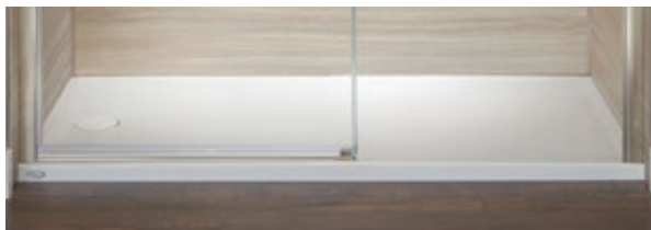
Concealed drain cover
